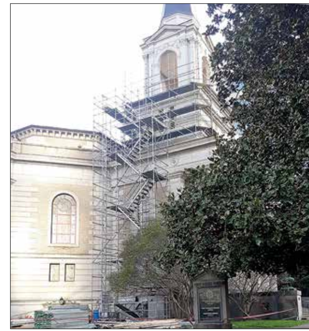
Knoxville's First Baptist Church is undergoing some repairs to the roof and steeple. Rev. Josh Gibson said the work there doesn't affect the chimes at all and work will be going on "for quite some time." Built in 1924 on West Main Street, the church is on the National Register of Historic Places. Photo by Mike Steely.
