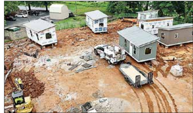
The first of Operation Hero's Hill's tiny homes are arriving at the Liberty Street complex. Twenty homes and a community center will welcome homeless veterans when the project is completed in August.
